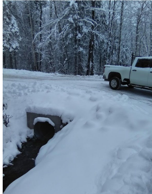
The culvert in segment 127132 was upsized using town funding after failing during the summer 2023 flooding.
