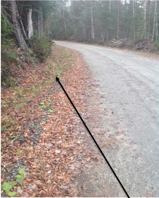
All segments have grader berms and poorly shaped shoulders, causing rill erosion.
